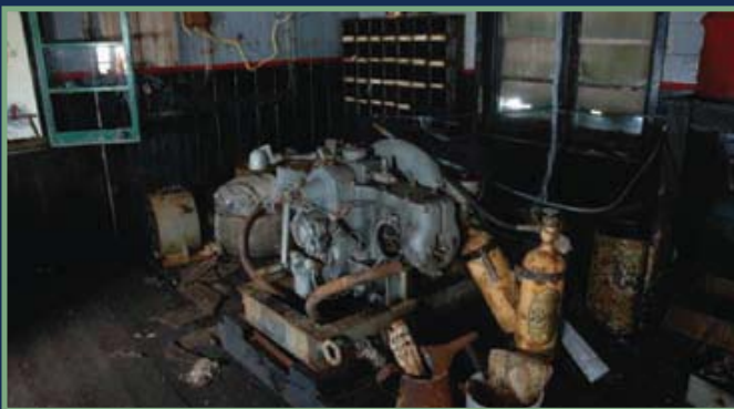
The Generator still in place in the Generator shed
